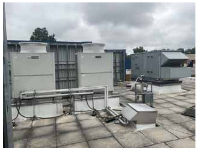
30 - ROOFTOP HVAC EQUIPMENT
