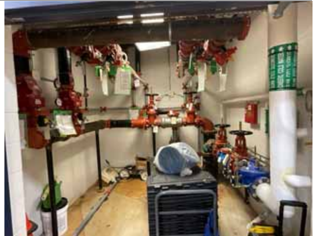
32 - DOMESTIC WATER/FIRE SPRINKLER ROOM
