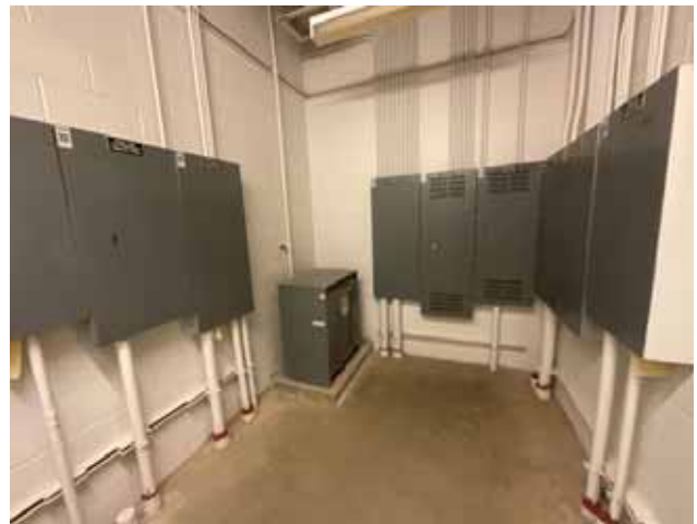
34 - 2ND FLOOR ELECTRICAL ROOM
