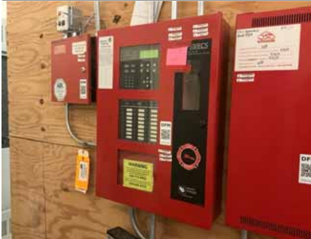
37 - FIRE ALARM PANEL
