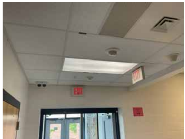
36 - FIRE ALARM SYSTEM
